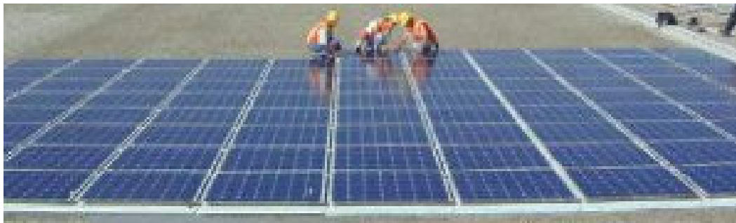
Powerlight flat roof system
